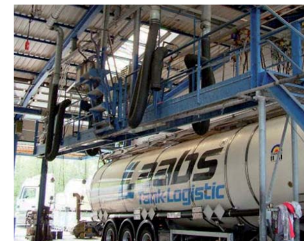
Two lane washbay for internal tanks
